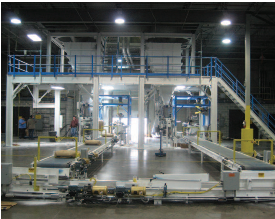
The two parallel packaging lines consistently fill up to 24 bags per minute, exceeding the company’s original packaging rate requirements.
